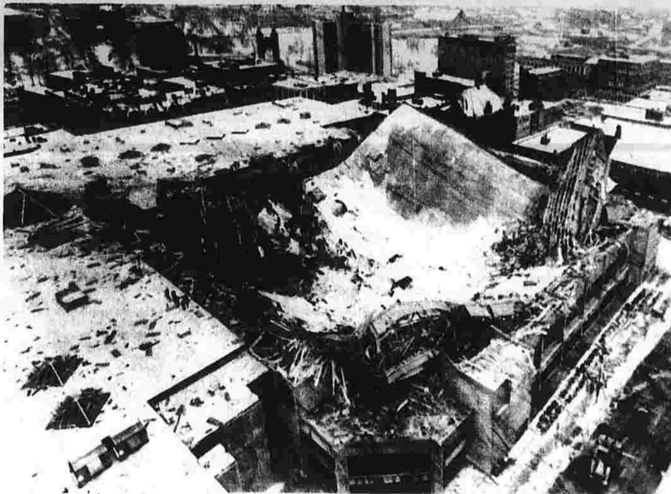
Cleanup crews moved in early this morning to start clearing away debris at the Hartford Civic Center. The massive roof caved in shortly after 4 a.m. today under tons of snow, ice and water. The cave-in happened only several hours after some 5,000 people had been in the center watching a basketball game. City officials and owners of shops in the center were stunned by the news and the thoughts of the economic impact it will have. (UPI photo)
