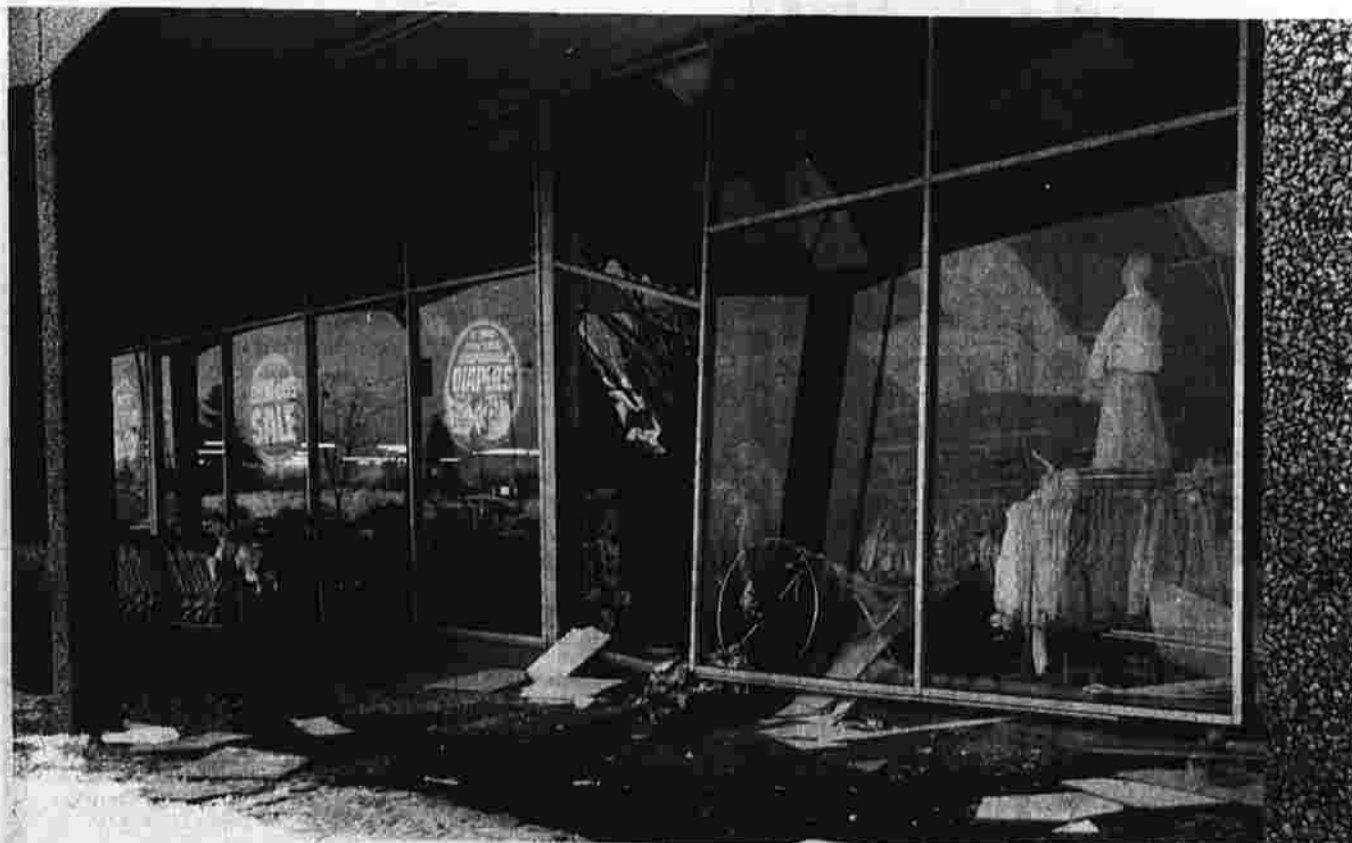
Light peeks through a hole in the collapsed roof of the K-Mart supermarket at 239 Spencer St. The roof caved in early this morning under the weight of snow and ice. (Herald photo by Pinto)
